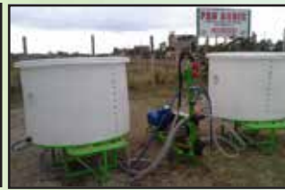
Central Spray Unit
