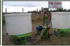
Central Spray Unit
